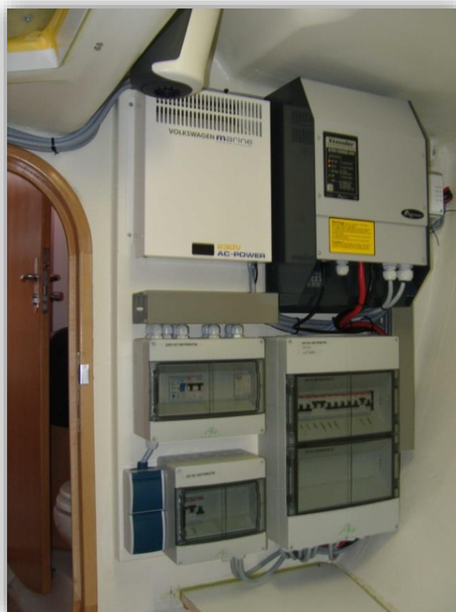
(Figure 5), Variable speed generator inverter and an Xtender
