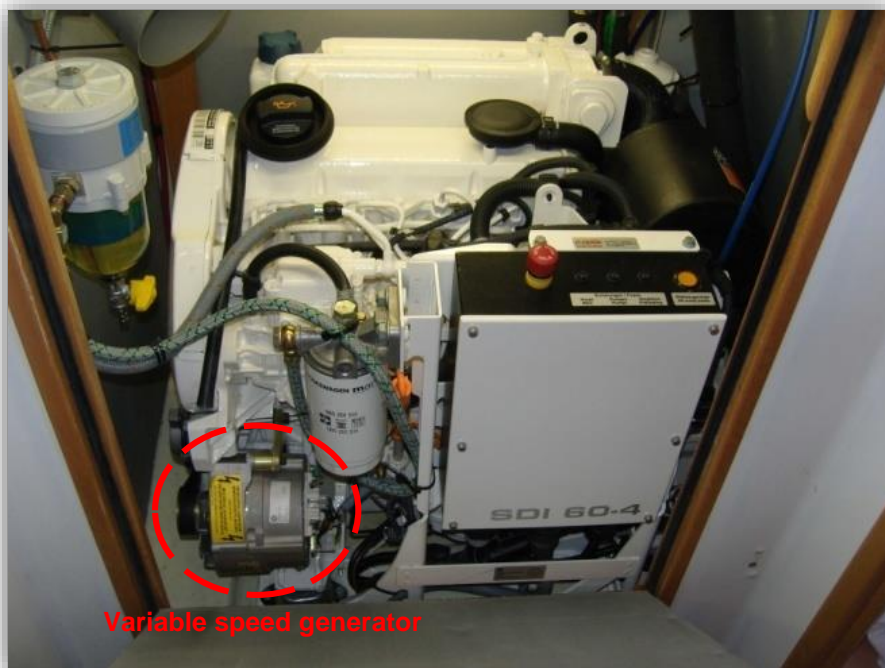
(Figure 4), Variable speed generator on a boat engine
